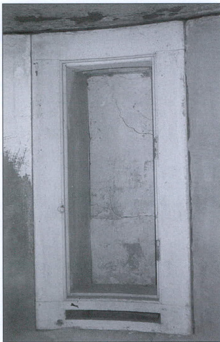
Door at the top of the weight shaft. Note the slot at bottom for the (missing) shelf. Photo by the author.
